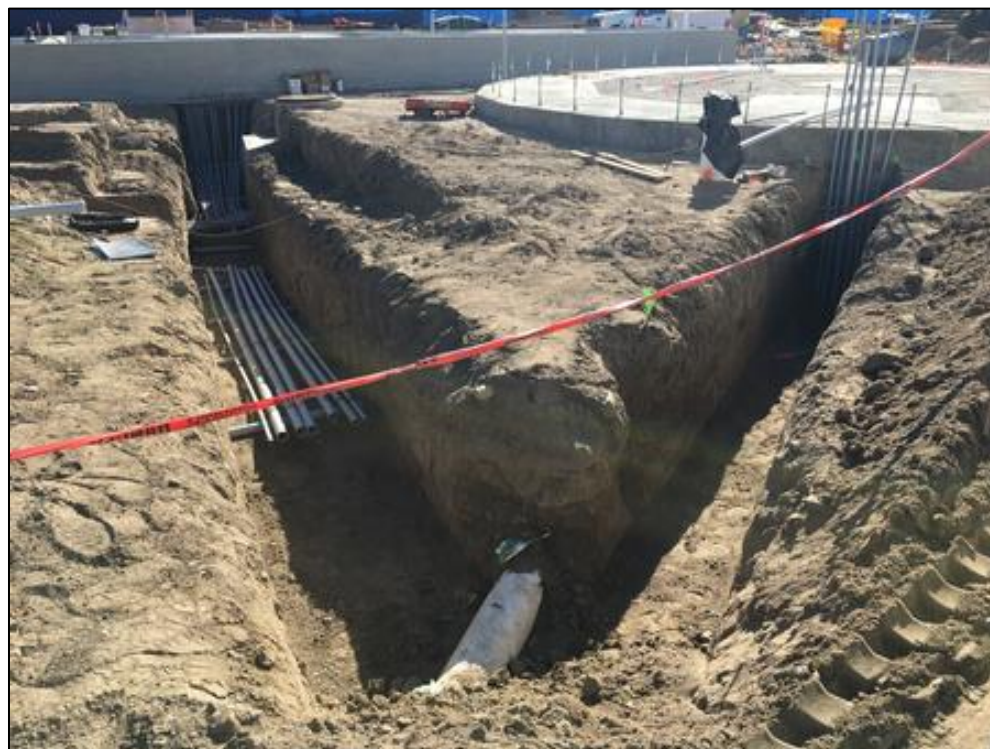
Electrical duct bank in digester area
