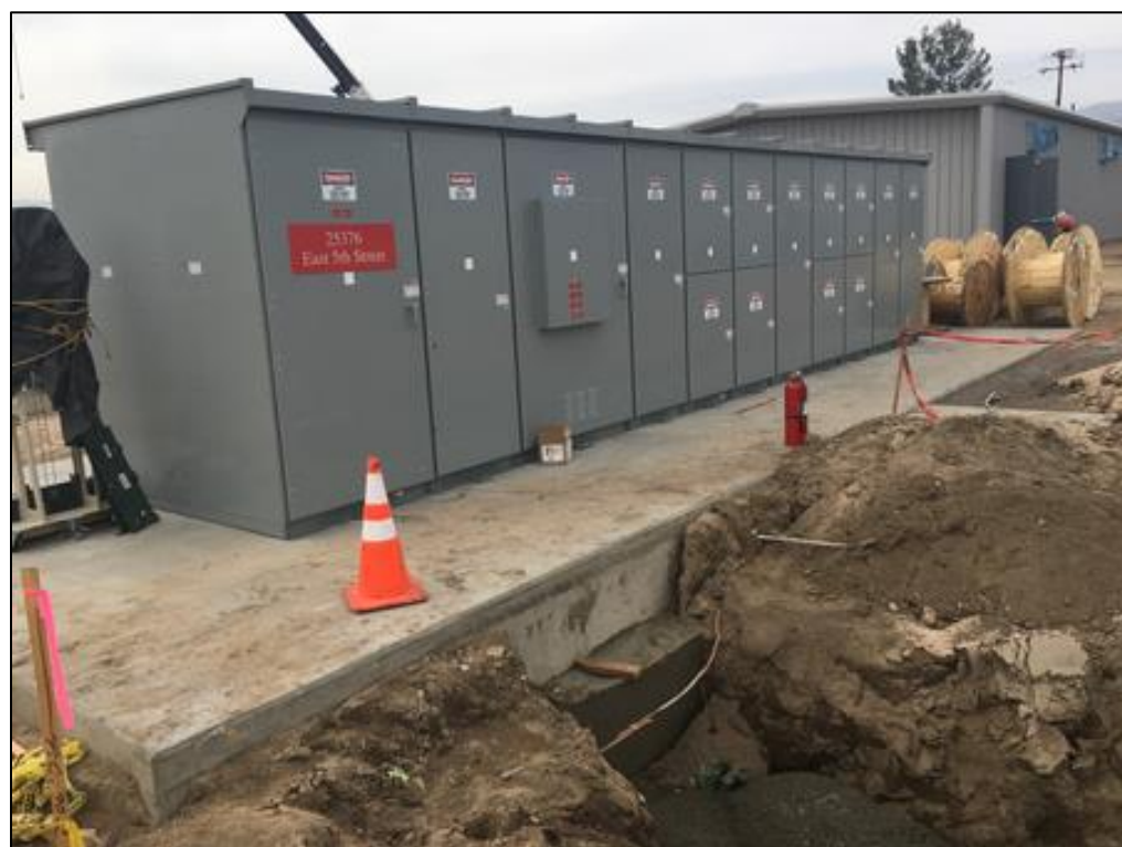
Electrical metering equipment
