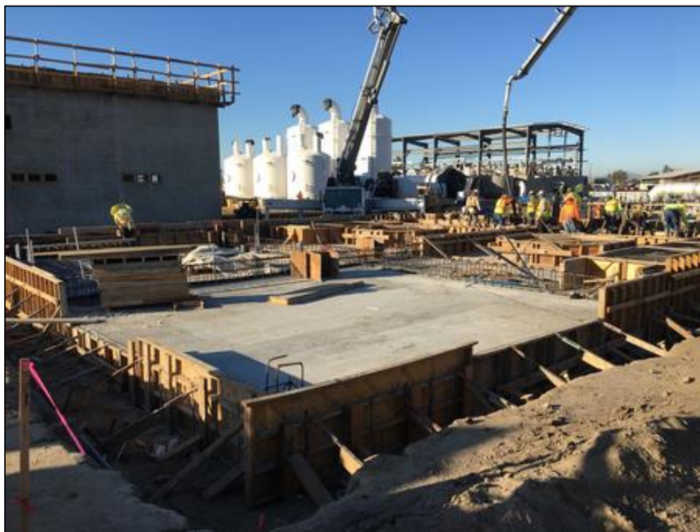
Chemical storage and metering facility
