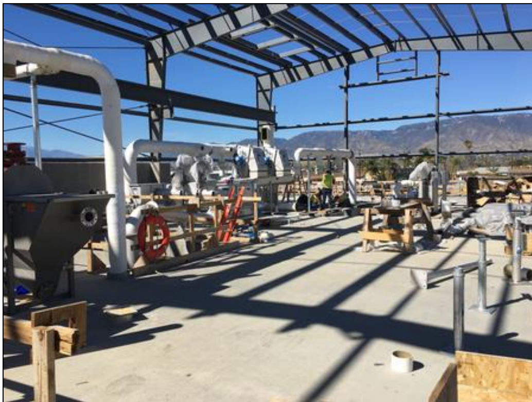
Inside of Headworks Building looking north
